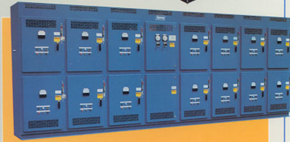
SCR power center for multi-zone control of float glass tin bath heating elements.
